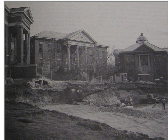
L.D.S. Campus being razed for the construction of the Church Office Building
